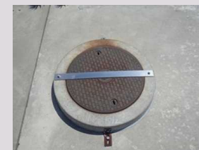
Manhole covers fastened down using metal bars (Unit 6&7)
