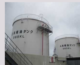
Light oil tanks for Unit 7 after replacement (Thickness of the steel plating of the tanks is approximately four times what it was)
