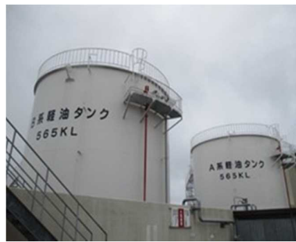
Light oil tanks at Unit 7
