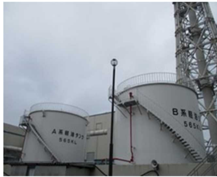
Light oil tanks at Unit 6
