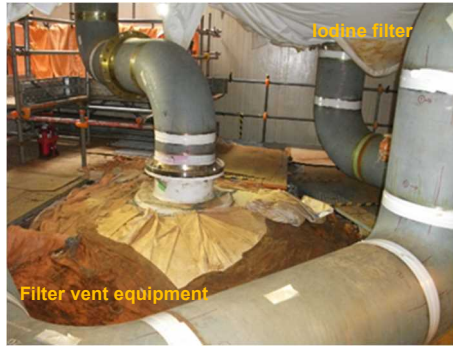
Pipes around iodine filter (Unit 6)
