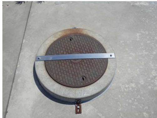
Anchored manhole cover
