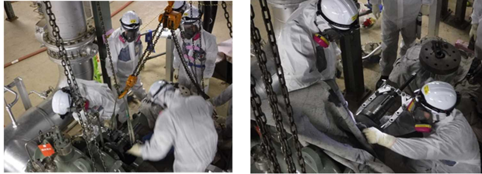
Training in disassembling pump bearings while workers wear full-face masks
