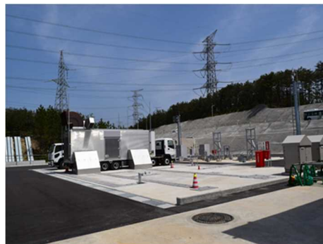
Additional air-cooled gas turbine power supply car
