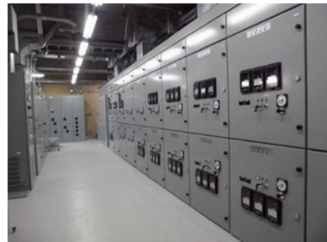
Emergency switchboard on the Arahama side
