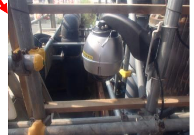
Drainage channel K/C pump (Monitoring camera)
