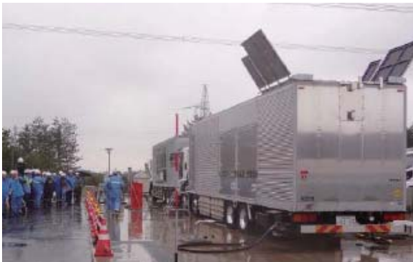
Start-up test for gas turbine generator vehicle
