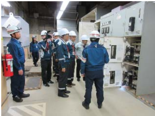
Power distribution panel submerged by tsunami (Unit 1)
