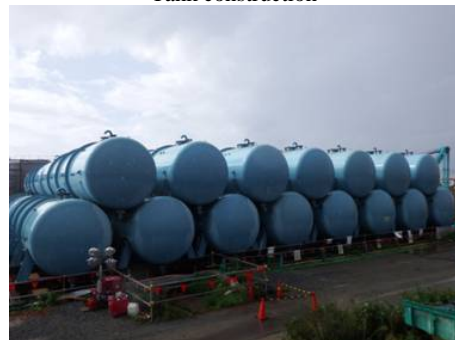
Storage of removed tanks
