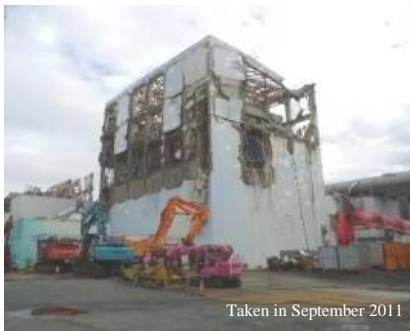
Prior to Debris removal
