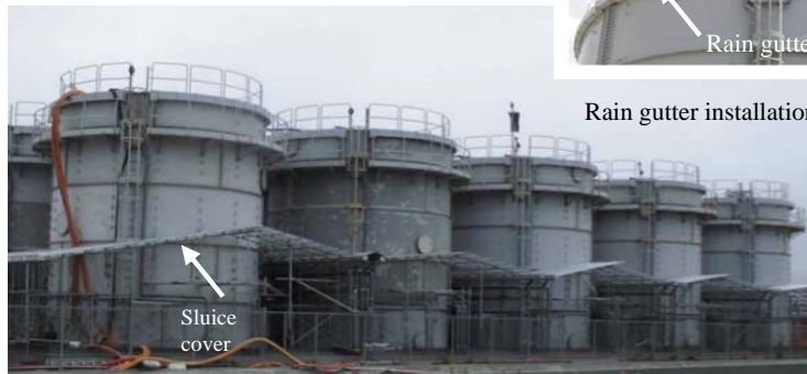
Rain countermeasures for tanks
