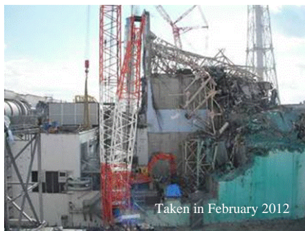
Prior to debris removal
