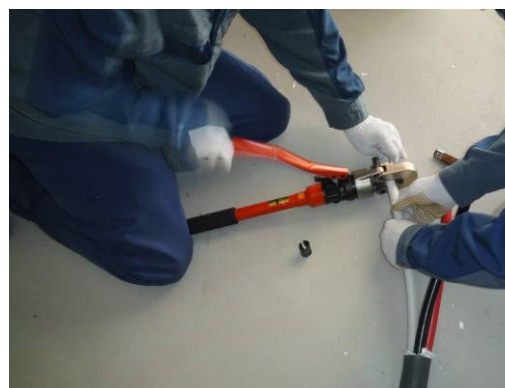
Training for handling low-tension cable terminals
