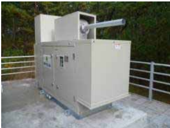
Monitoring post back-up generator
