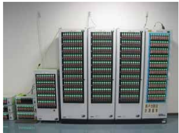
Alarm person dosimeters: 120→500 units (Anti-seismic building)
