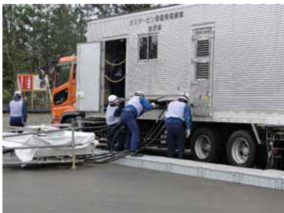
Training in supplying power using GTG
