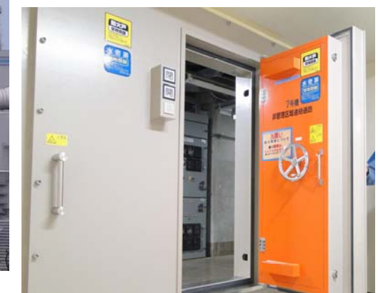
Water-tight door : Preventing flooding of critical areas (about 60 places)
