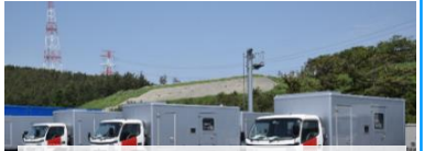
Gas turbine generators/power supply trucks
