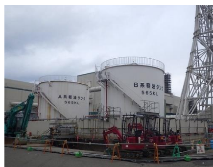
Unit 6 diesel tank
