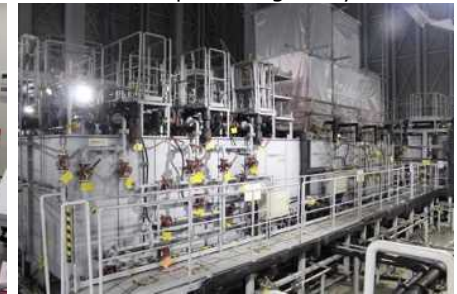
Additionally installed ALPS
