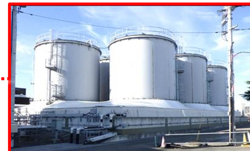
J8 area tanks
