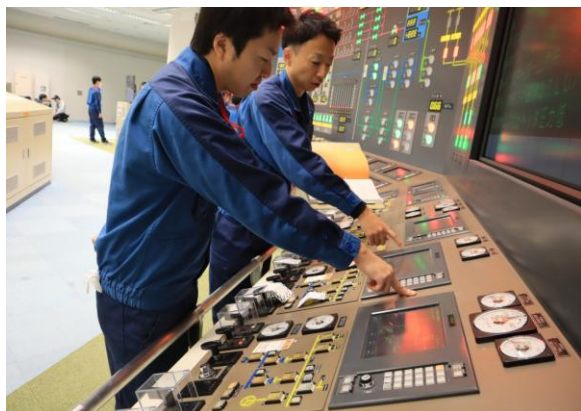
Operations instructions in the main control room
